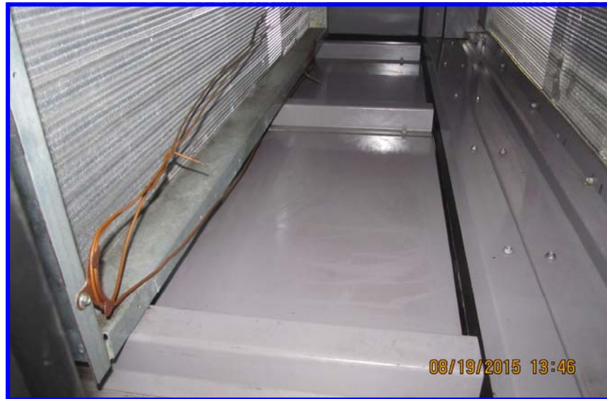
MECHANICAL ROOM # 1- AHU ON RIGHT PAN
