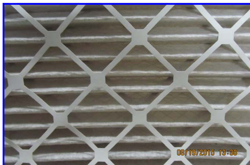
MECHANICAL ROOM # 1AHU ON RIGHT – FILTER
