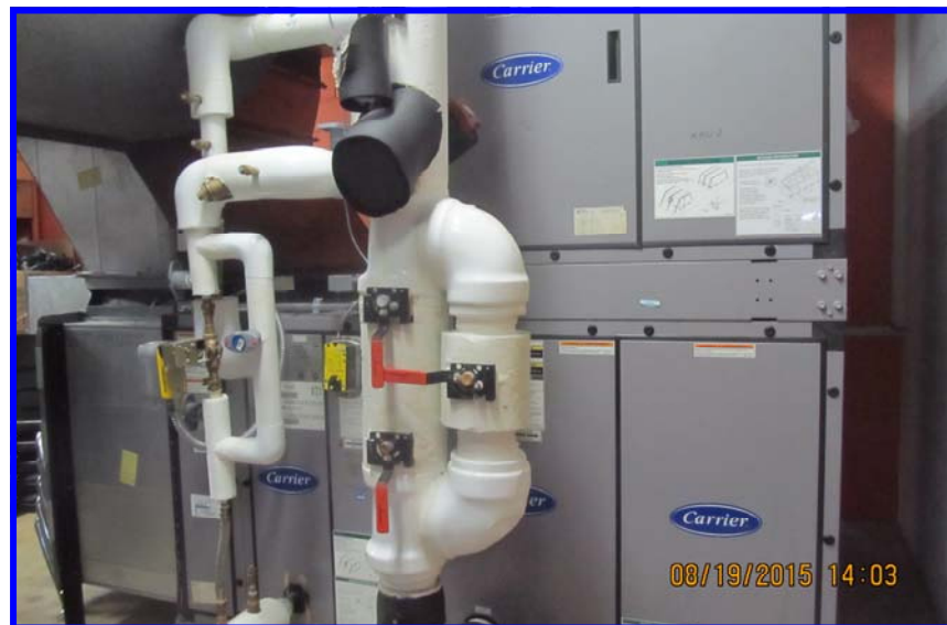
AHU #3 MECH ROOM
