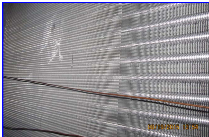
MECHANICAL ROOM # 1 AHU LEFT - COIL
