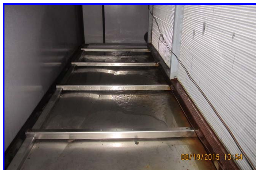
MECHANICAL ROOM # 1 AHU ON LEFT- PAN
