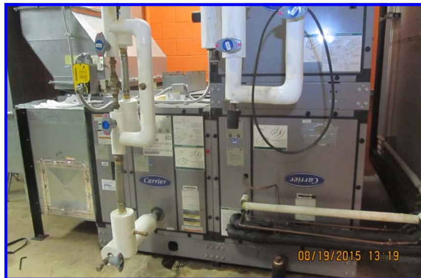
MECHANICAL ROOM # 1 AHU ON RIGHT
