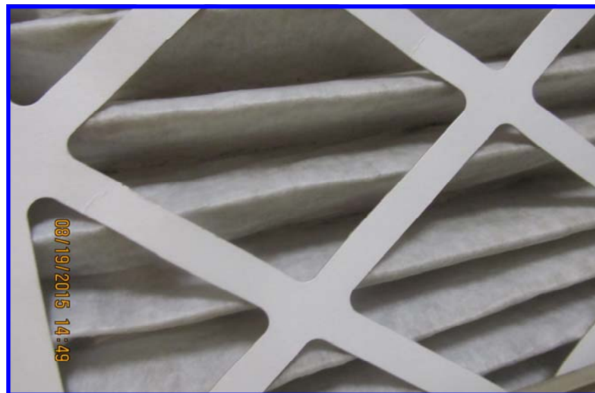
UNIT FOR ROOM #407 -FILTER
