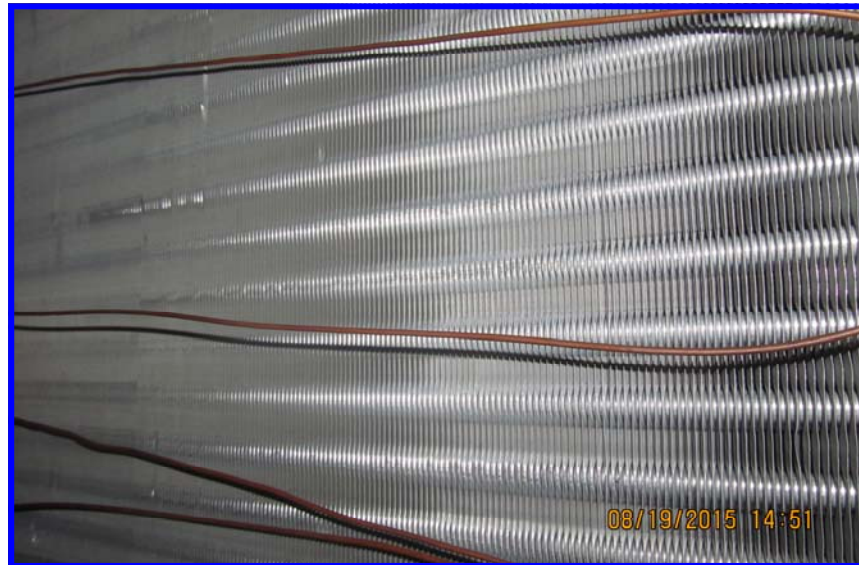
UNIT FOR ROOM #407 COIL
