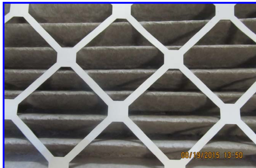
MECHANICAL ROOM # 1AHU ON LEFT- FILTER
