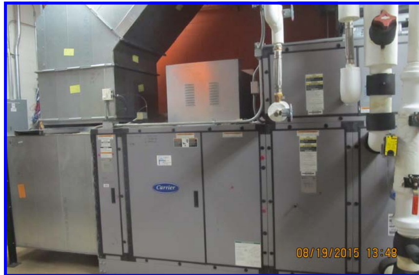
MECHANICAL ROOM # 1 AHU LEFT MECH ROOM- PAN
