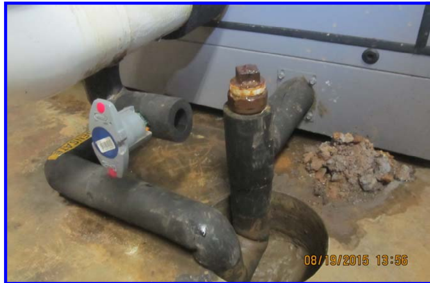
MECHANICAL ROOM # 1 AHU LEFT - TRAP
