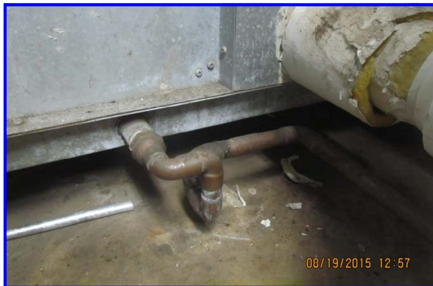
AHU #9 PAN UNABLE TO ACCESS
