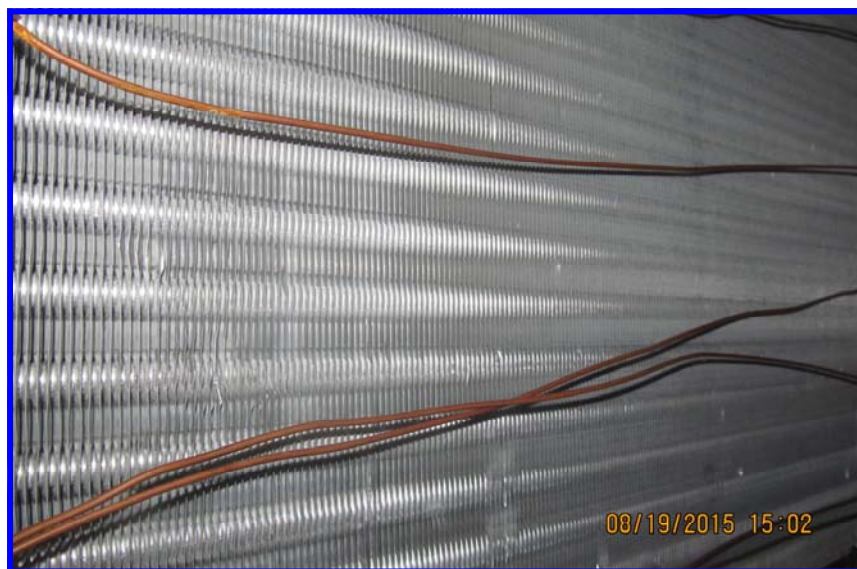
UNIT FOR ROOM #405- COIL
