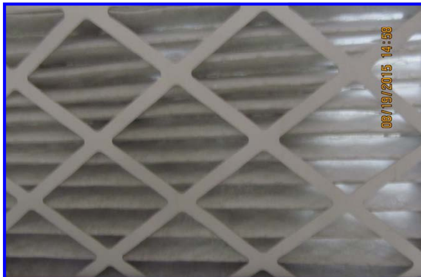
UNIT FOR ROOM #405- FILTER
