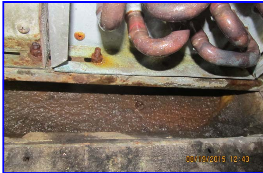
AHU #10 PAN VERY DIRTY
