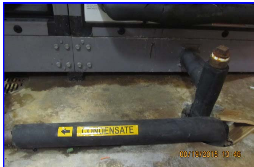
MECHANICAL ROOM # 1AHU ON RIGHT- TRAP
